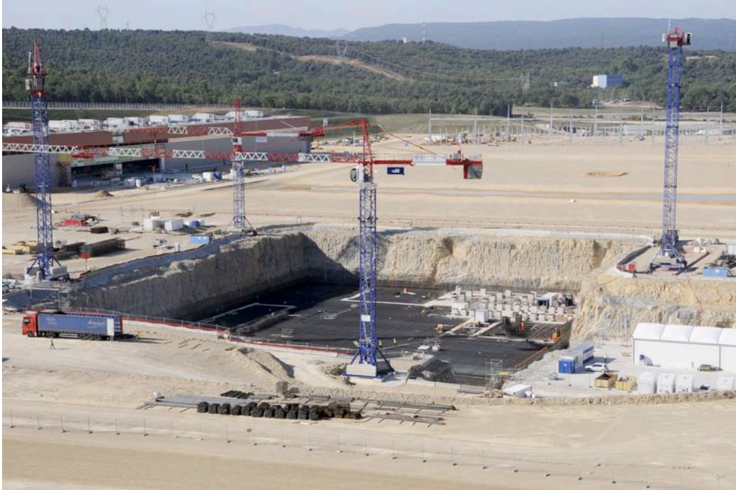
Looking south over the Tokamak Complex Seismic Isolation Pit in September 2011. Photo: Altivue/ ITER Organization .
