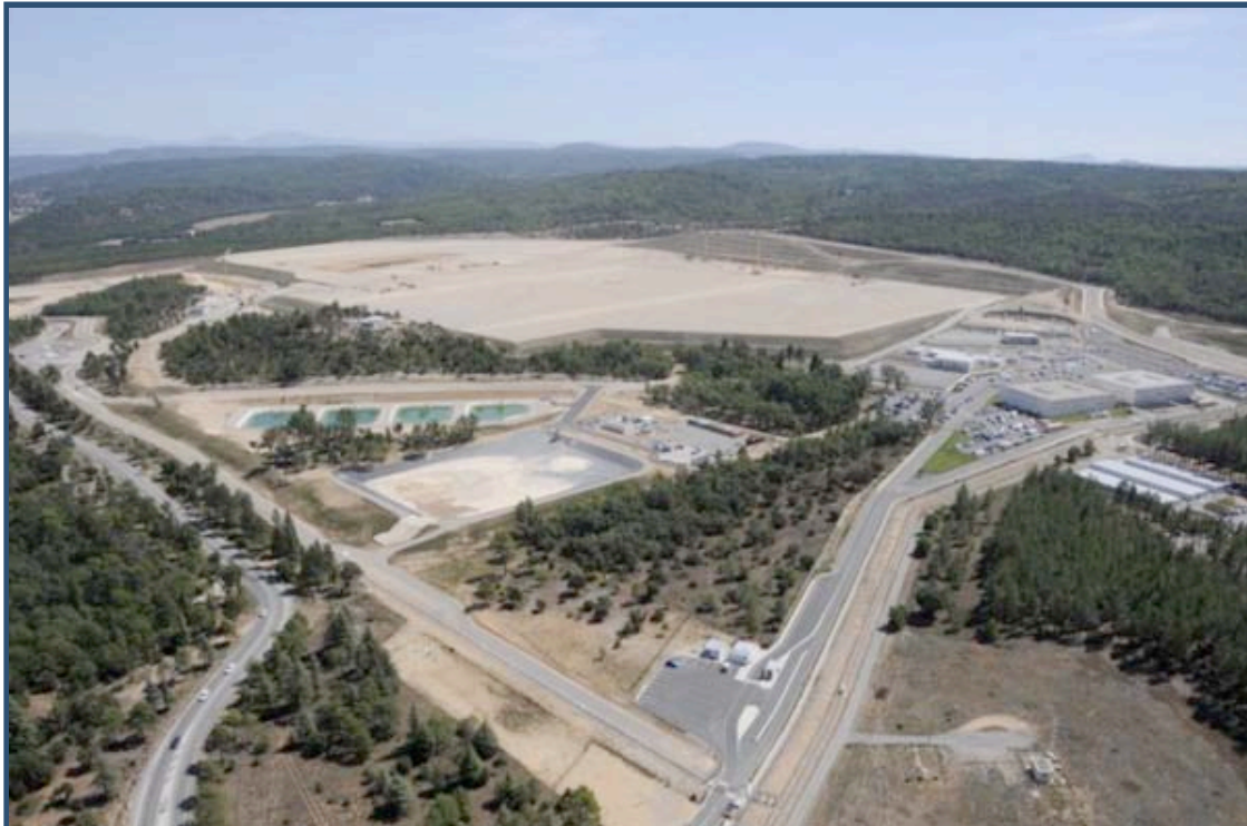
Aerial view of the ITER site as of September 2010 (courtesy of ITER Organization)
