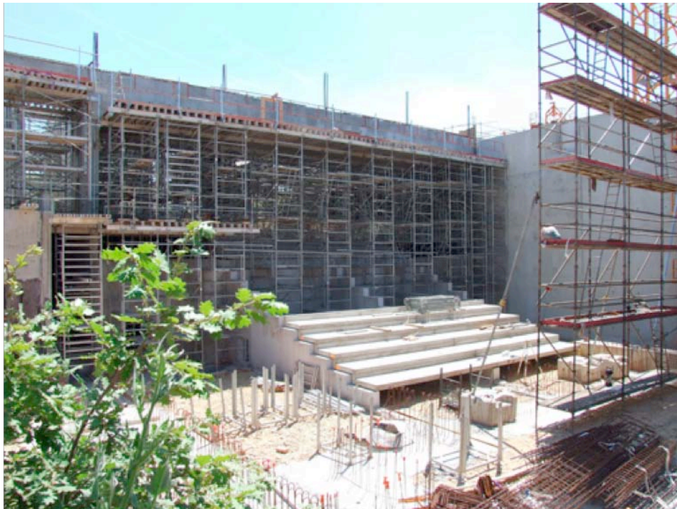
Future amphitheater in the ITER office building (photo courtesy of ITER Organization)
