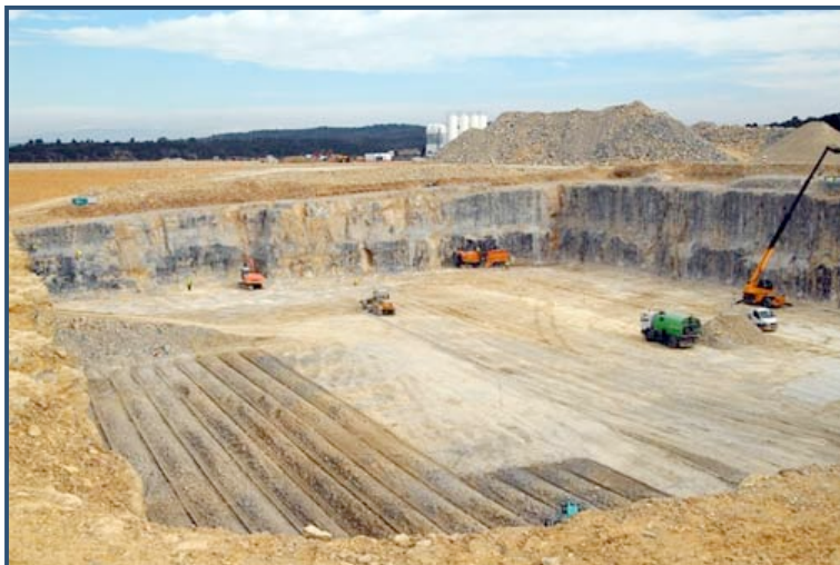
Excavation for the future Tokamak Complex Seismic Isolation Pit (photo courtesy of ITER Organization)
